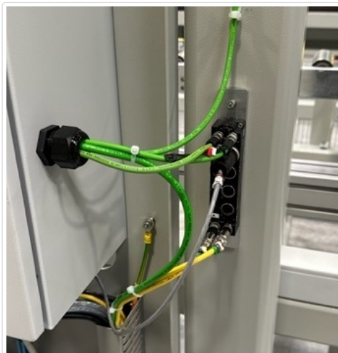
Analogue Fieldbus box next to infeed electrical panel
